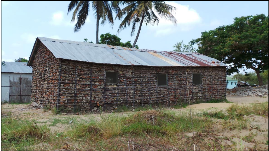
Figure 40: External structure of a local church made of mangrove wood (Chinde Headquarter) [Díaz P., I.; Oct. 2017].
