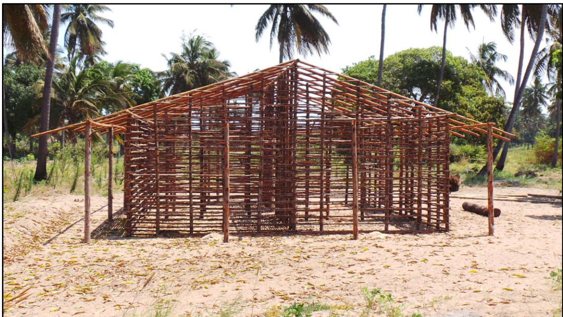
Figure 39: A house frame built with Ceriops tagal poles (Village of Pambane) [Díaz P., I.; Oct. 2017].
